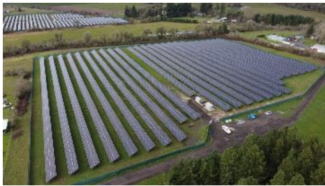
Red Prairie Community Solar project in Oregon
