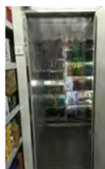
A curtain installed in a walk-in refrigerator
