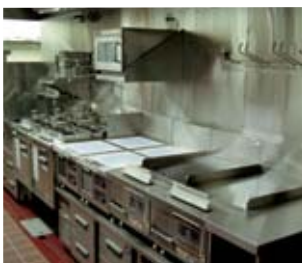
Electric kitchen equipment that reduces energy use and CO 2 emissions
