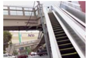
Escalator running next to the steps
