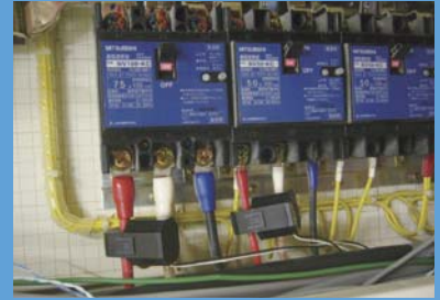
Smart sensors (power consumption measuring instruments used for visualization of power use)
